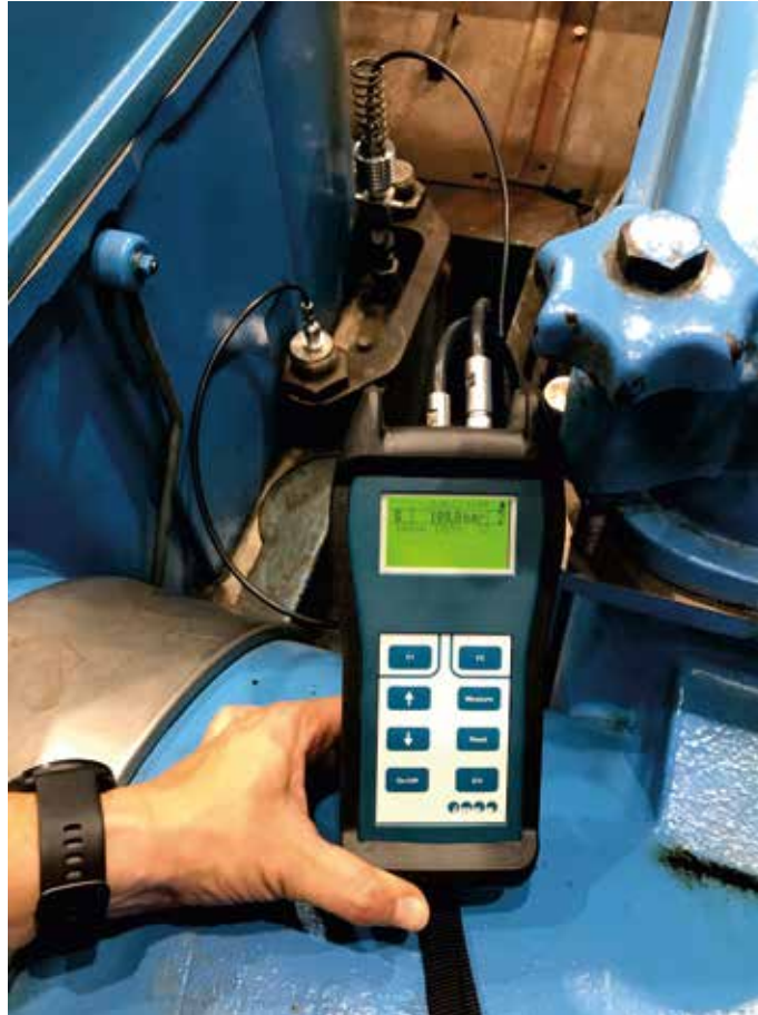
EPM-XP plus-vibro installed on a MAN 12V 48/60 engine at the Endesa powerplant in Melilla
