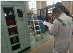
Control cabinet checking
